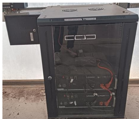
Figures 7 and 8. Proconsult inverters and batteries
