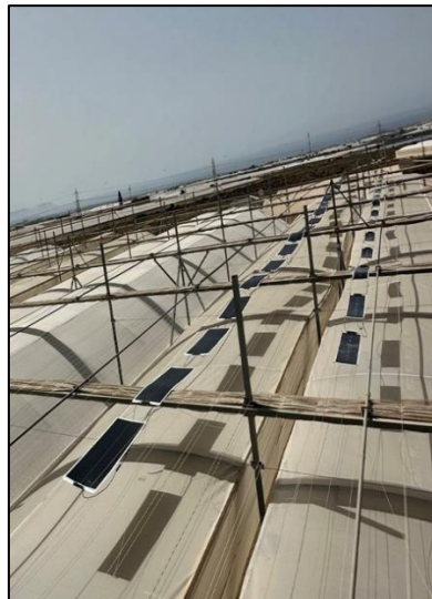
Figures 3 and 4. Two rows of Energy Glass Photovoltaic panels covering 4.12% of the total greenhouse roof area.
